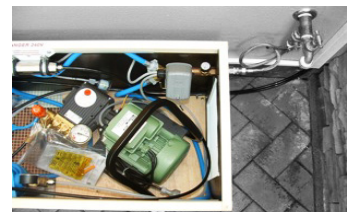
Pump detail & water connection
